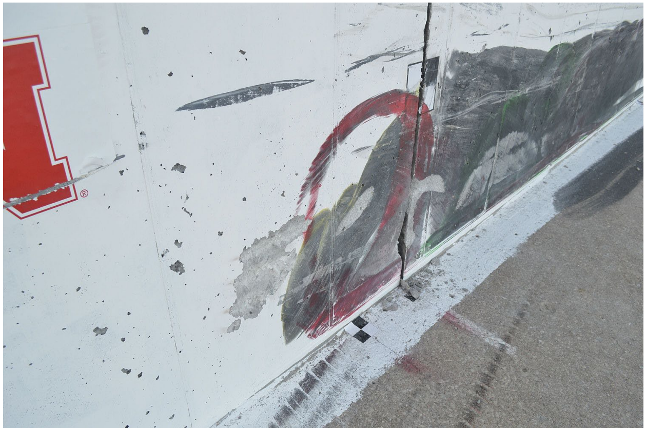
Figure 6.13 System Damage Near Expansion Joint, Test No. MTL6-1
