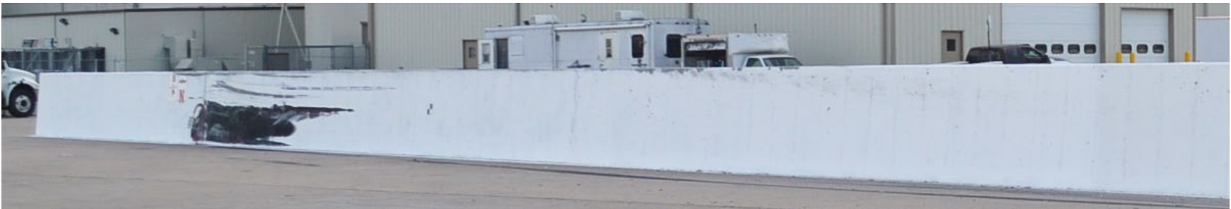
Figure 6.11 System Damage, Test No. MTL6-1
